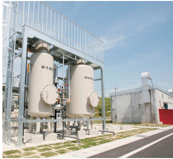
Waste water discharge treatment facility
