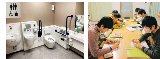
We have formulated a three-year plan to improve the workplace environment, and are making systematic improvements such as installing restrooms with consideration of people with disabilities
