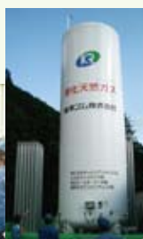
Liquefied Natural Gas tank
