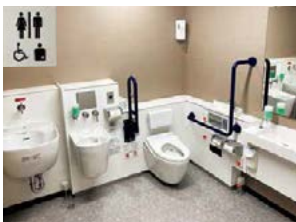
We have formulated a three-year plan to improve the workplace environment, and are making systematic improvements such as installing restrooms with consideration of people with disabilities
